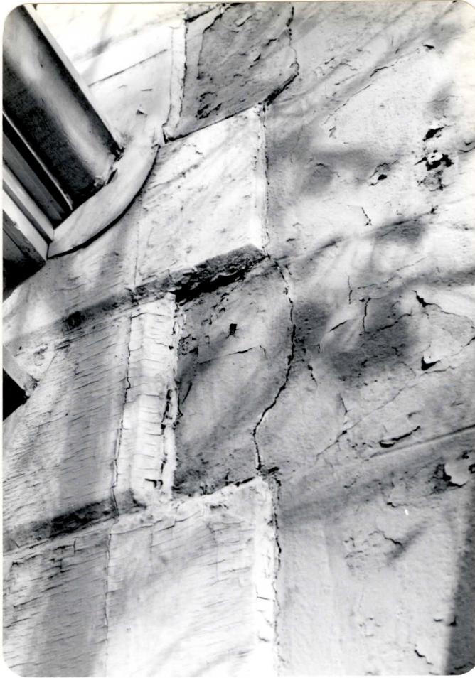
Figure 73. View of quoins, west wall, showing present condition and, right, minor cracks in roughcast.
